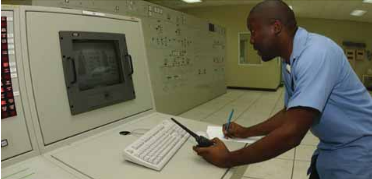
Smart grid sensors and controls and well-trained technicians enhance operating efficiency of the electric grid in The Bahamas
